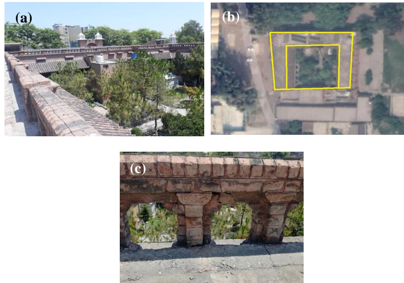
Fig. 4. (a) Irregular Shape (b) Rectangular Shape (c) Eroded and Non-Restrained Parapet Walls
