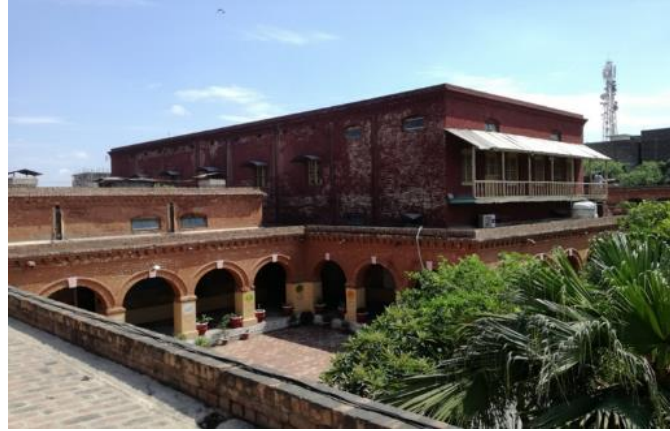
Fig. 10. Parapet Walls Not Restrained to the Roof and Fallen on the Left Side
