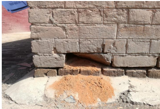
Fig. 11. Eroded Wall of Building Room
