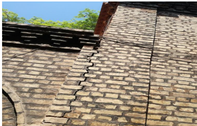
Fig. 12. Wide Crack Between Veranda and Building Room
